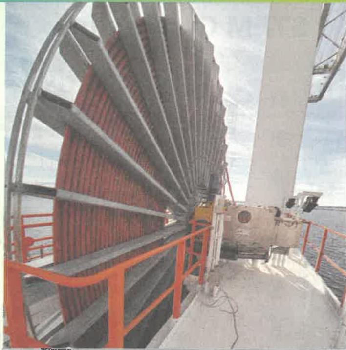
This shore-power cable reel provides 13,200 V of electricity to the crane.
